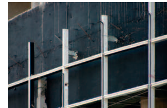
Figure 8.9 Water vapor retarder applied to the outside of a building envelope, detailed view, Dubai (UAE)
