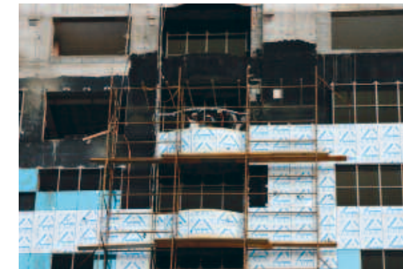
Figure 8.8 Water vapor retarder applied to the outside of a building envelope, bituminous coating on concrete, Dubai (UAE)
